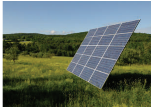
Solar photovoltaic panels that automatically track the sun’s movement greatly increase electrical generating capacity.
